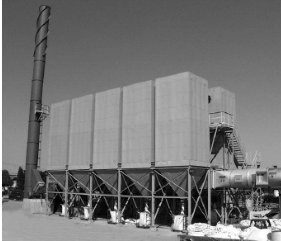
Figure 4—Bag House (Pollution Control Equipment).
